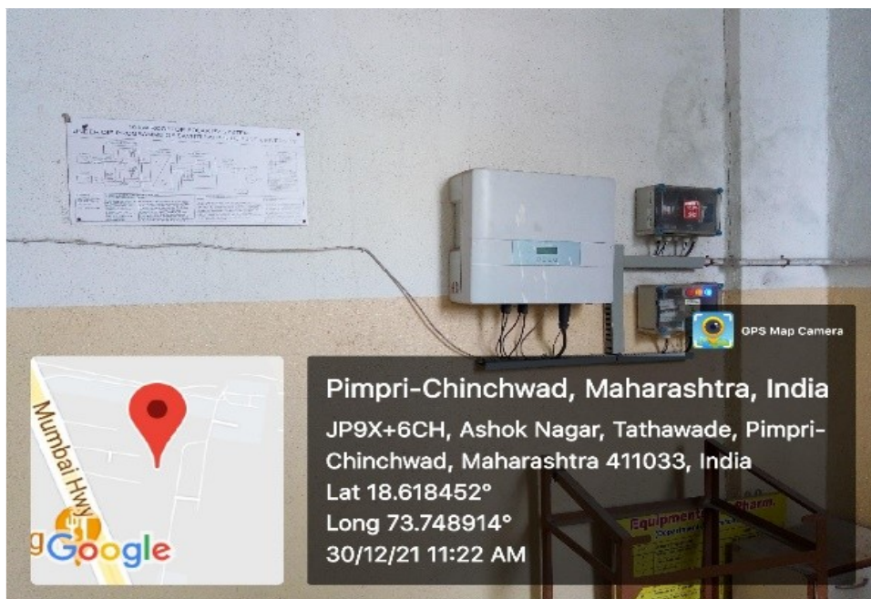
Wheeling to the Grid
